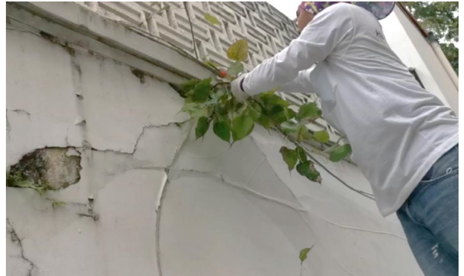
Removal of aggressive plant root underneath the paint
